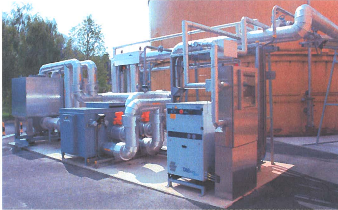
Photo 3: Biogas purification station; © Van der Wiel bv)
